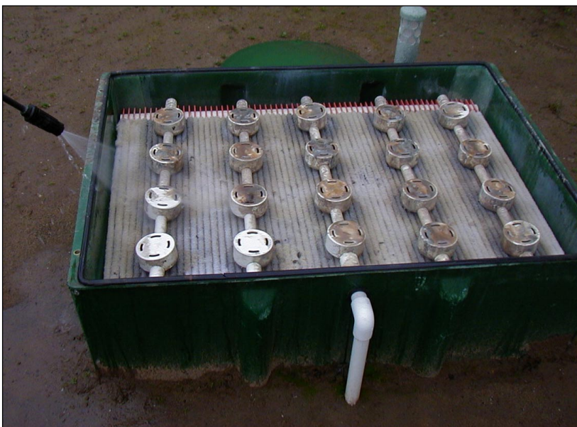
Figure 9: Typical servicing of AdvanTex textile medium. (An underdrain valve is opened during a filter washdown that allows sloughed solids to flush back into the process tank, so there is no removal or wasting of media.)
