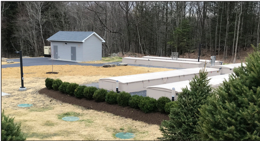
An AdvanTex® AX-Max™ Wastewater Treatment System – with its low life-cycle costs and small footprint – was chosen as the best replacement for a failing treatment plant in the community of Pinebrook. (Photo courtesy of the Dutchess County Water and Wastewater Authority.)
