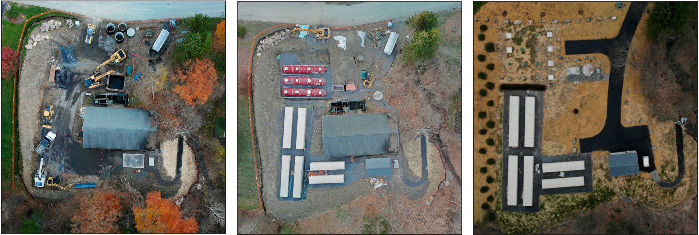
Between November and April, six AdvanTex AX-Max units were installed to replace Pinebrook's failed rotating biological contactor (RBC). The final photo on the right shows that the RBC and the building once housing it have been removed. (Photos courtesy of the Dutchess County Water and Wastewater Authority.)
